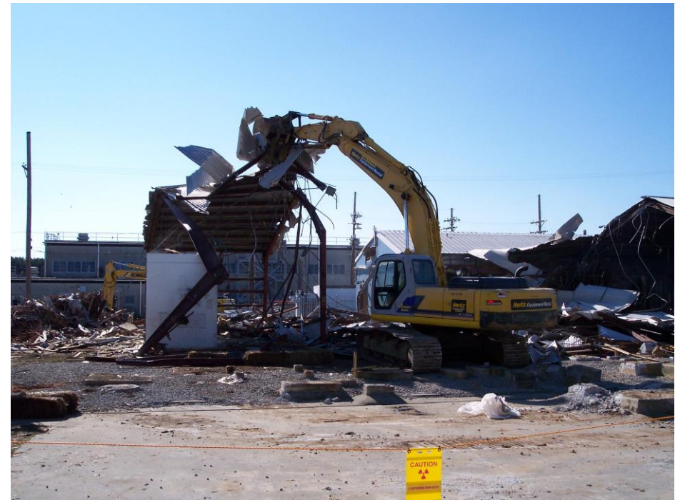
CEG Personnel Performed the First DOE Complex Open-Air Demolition of a Hot Cell
